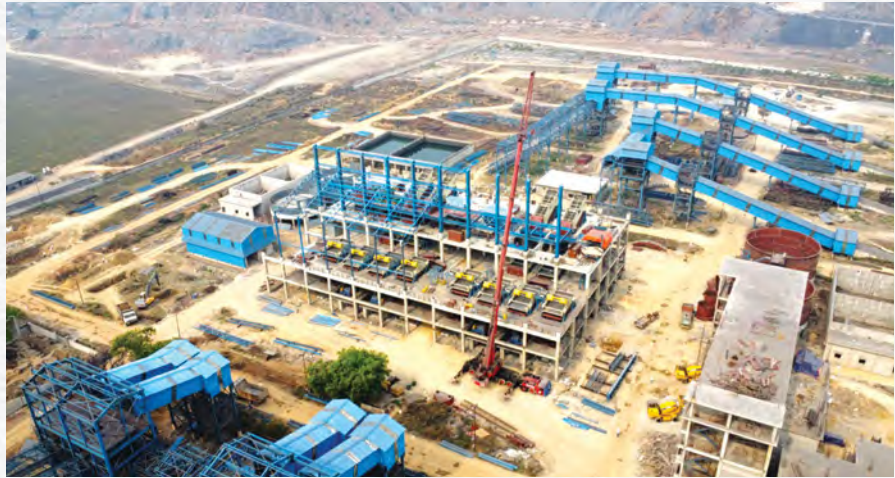
IB-Valley Washery (10.0 Mtpa capacity) at Lakhanpur
