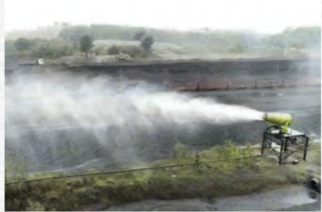
Trolley Mounted Fog Cannon (100 m throw) installed at Belpahar OCP
